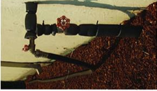
Properly insulated pipe
